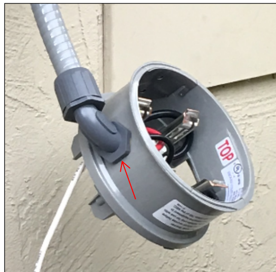
Figure 7. Point of Interconnection
